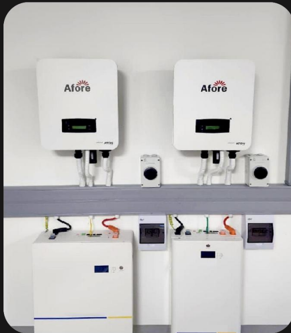
Country: South Africa Product: Single Phase Hybrid Inverter 6kW Battery: 11kW·h
