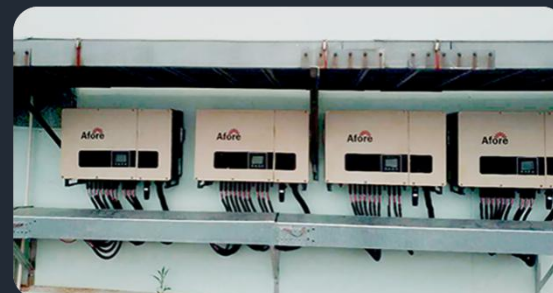
Product: Three-phase 60kW Project Size: 500kW
