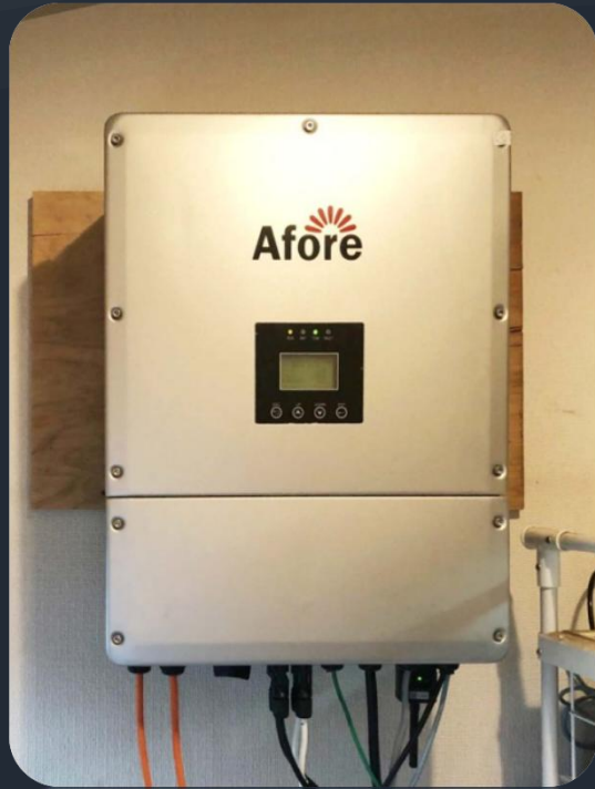
Country: Japan Product: Hybrid Inverter 6kW Project Size: 6kW
