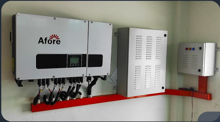
Country: Malaysia Product: Three-phase 60kW Project Size: 85kW
