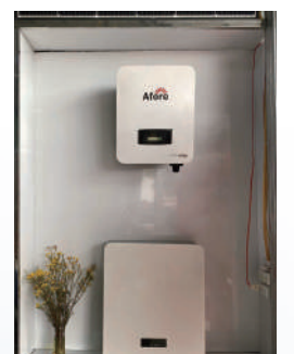
6kW Battery: 10kW-h Vietnam
