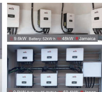
9.6kW Battery: 52kW-h 48kW Jamaica
