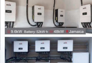
9.6kW Battery: 52kW-h 48kW Jamaica
